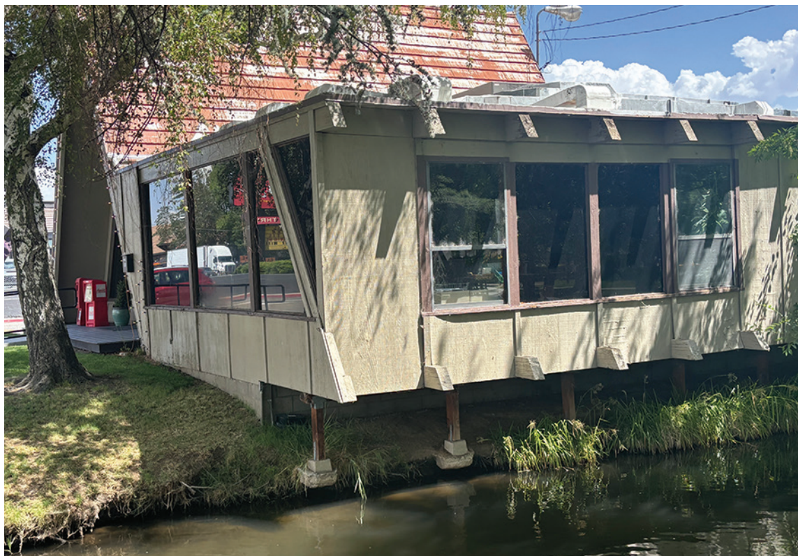
Bishop Chamber building. Notice the footings suspended in midair...
