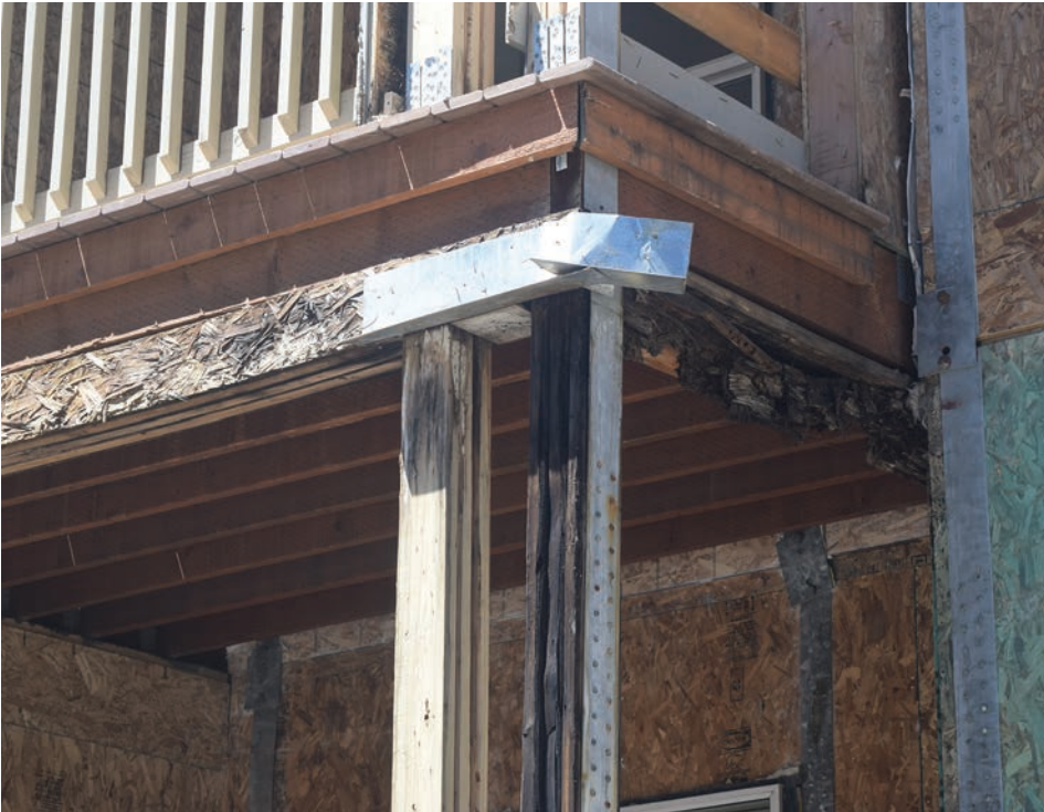
Some of the damage on the building revealed once the siding was removed
